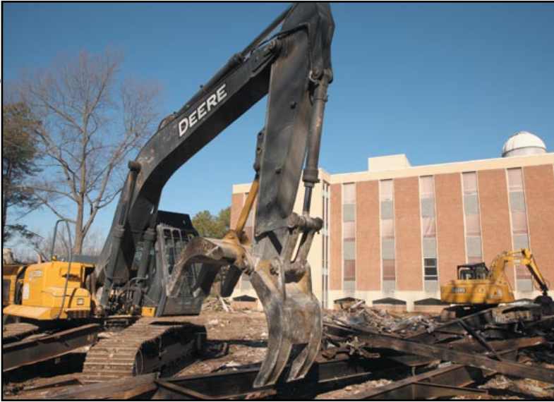
Although its operating budget is tight, William and Mary presses on with an ambitious new building program.
